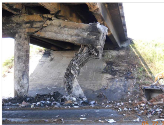
Figure 2. Resulting damage caused by the tractor-trailer collision with the SC Highway 150 bridge over I-85 (Kudelka 2011)
