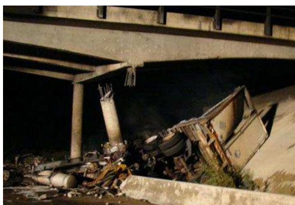
Figure 1. Pier support failure caused by tractor-trailer impact in Grand Junction, CO (Gallegos and McPhee 2007)
